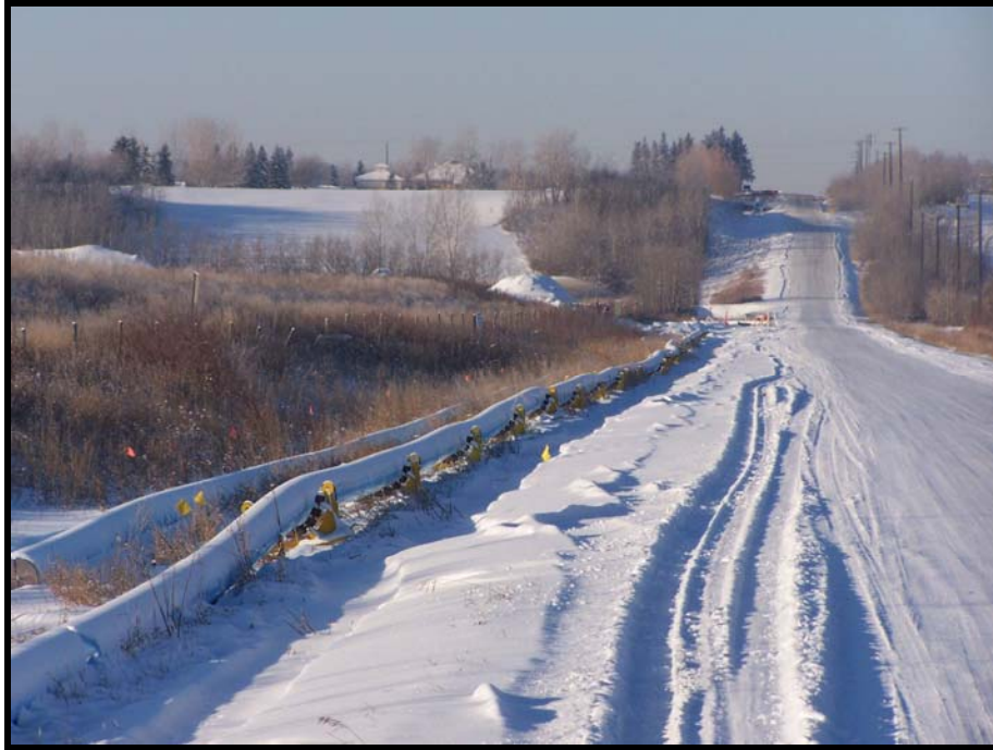
Figure 2. 153 Ave NE Road Right of Way Showing Fused PVC Pipe on Rollers
