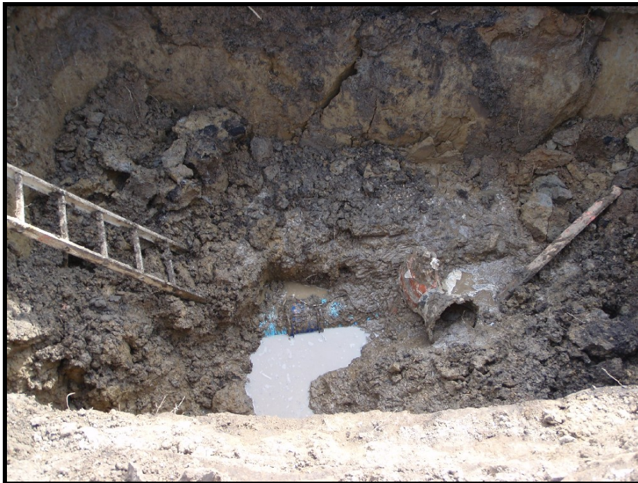
Figure 6. Leaky valve at 153 Ave NE
