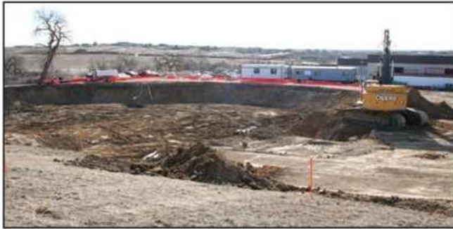
First work on Phase 2 at Broomfield WRF involves excavating for construction of new secondary clarifiers. Salida-based Moltz Construction Inc. is the general contractor.
