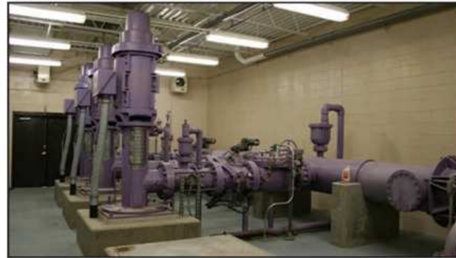
New pump station at Broomfield's water reclamation plant was completed in 2003 along with distribution pipelines to provide non-potable water for direct irrigation reuse or storage at Great Western Reservoir.
