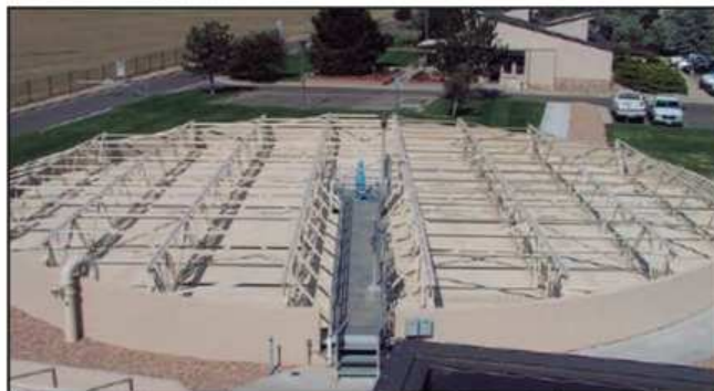
Grit removal, above, and new, covered clarifier. Existing basins will be covered during Phase 2 as odor control efforts will become complete.
