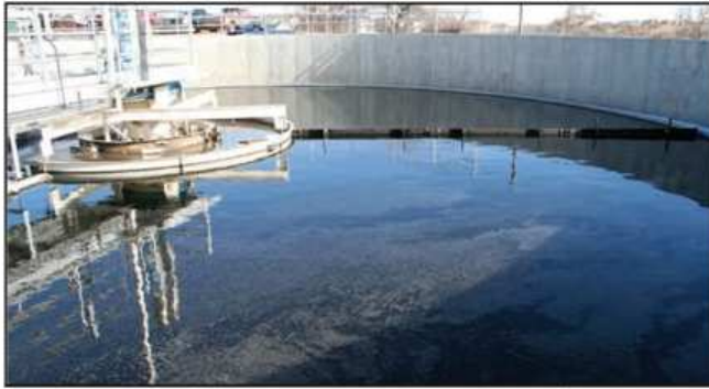
Two new secondary clarifiers were constructed during Phase 1 of improvements to the Broomfield Wastewater Reclamation Facility. Phase 2, with expected completion in 2010, will add two more. Clarifiers separate the active sludge biomass from the secondary effluent through settling while oil and other floating contaminants are skimmed from the surface.
