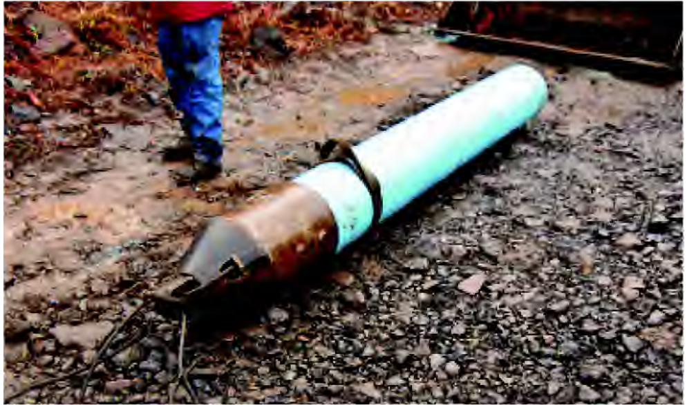
Figure 3: By pulling this "prover" through the host pipe, it demonstrated that both the pipe and pulling head could negotiate the entire run.
