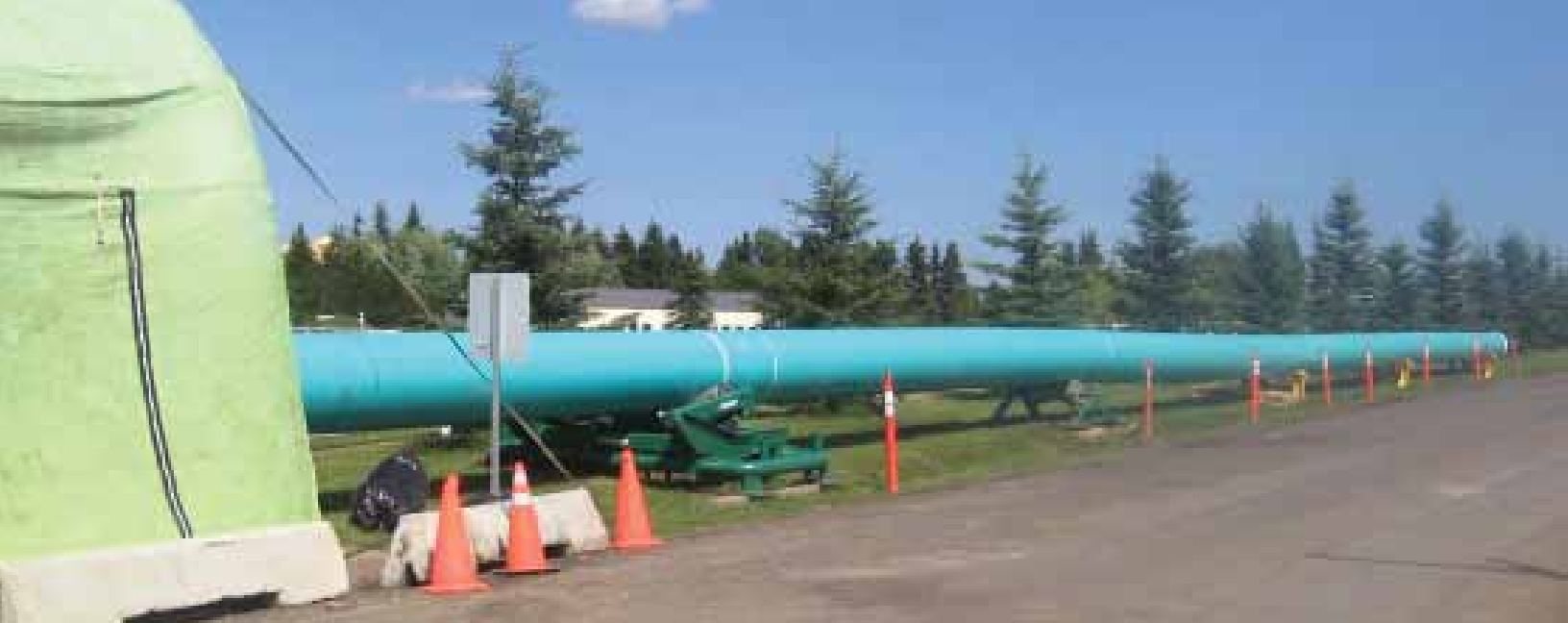
Fusible Brute PVC pipe ends and fusion machinery are sheltered during the installation
