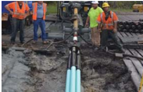
Tideland Electric Cooperative Bellhaven, NC
