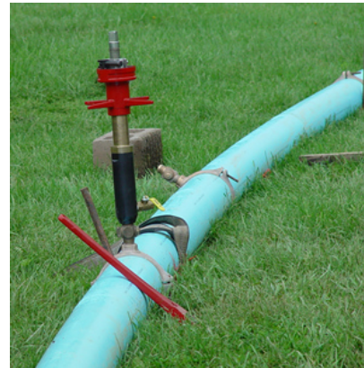
Standard PVC tapping saddles were installed and taps were performed using a standard PVC tapping machine with PVC cutting bits. The first set of taps was done on an empty line following Uni-Bell tapping procedures, replicating a new installation. The second set of taps was done on a full line at 150 psi, simulating the addition of a service tap to an active line (wet-tap).
