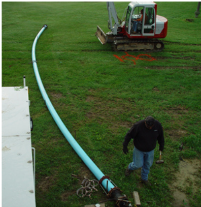
A 60-foot length of 6" DR18 Fusible C-900® with two fused joints was positioned to the recommended radius of 144 feet. Three quarter-inch saddles and corporations were used.
